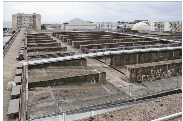
New ramp leading to the roof of the submarine basis at Saint-Nazaire, France, and the new outlook that becomes iconic for the district (Project by Manuel de Solà-Morales).
